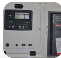
Control Panel & MCB
